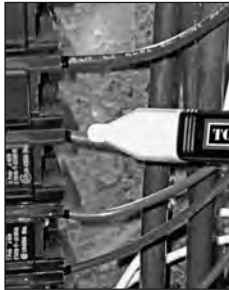
AC Voltage in junction boxes
